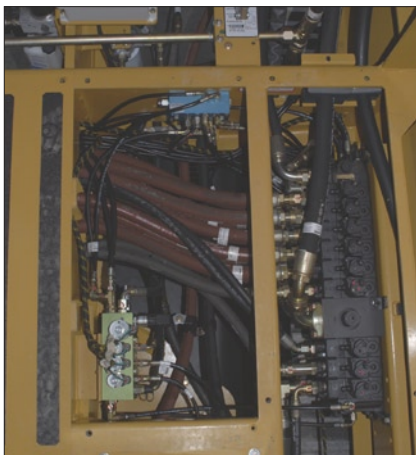
All valves are easily accessed under the walk-up platform
