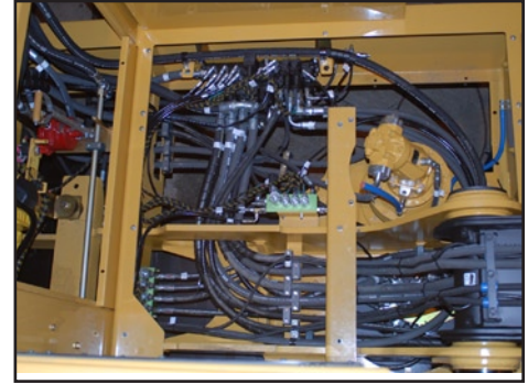
All valves are located underneath the walk-up platform
